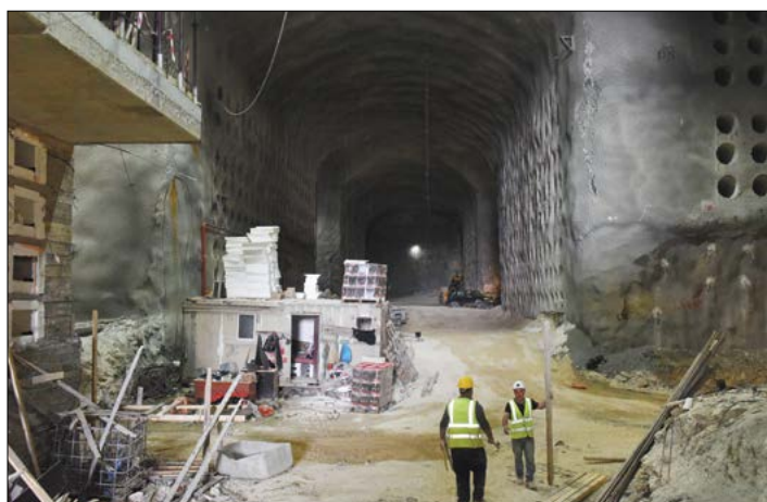
Workers carry materials in the tunnels where the underground cemetery project is being built.
